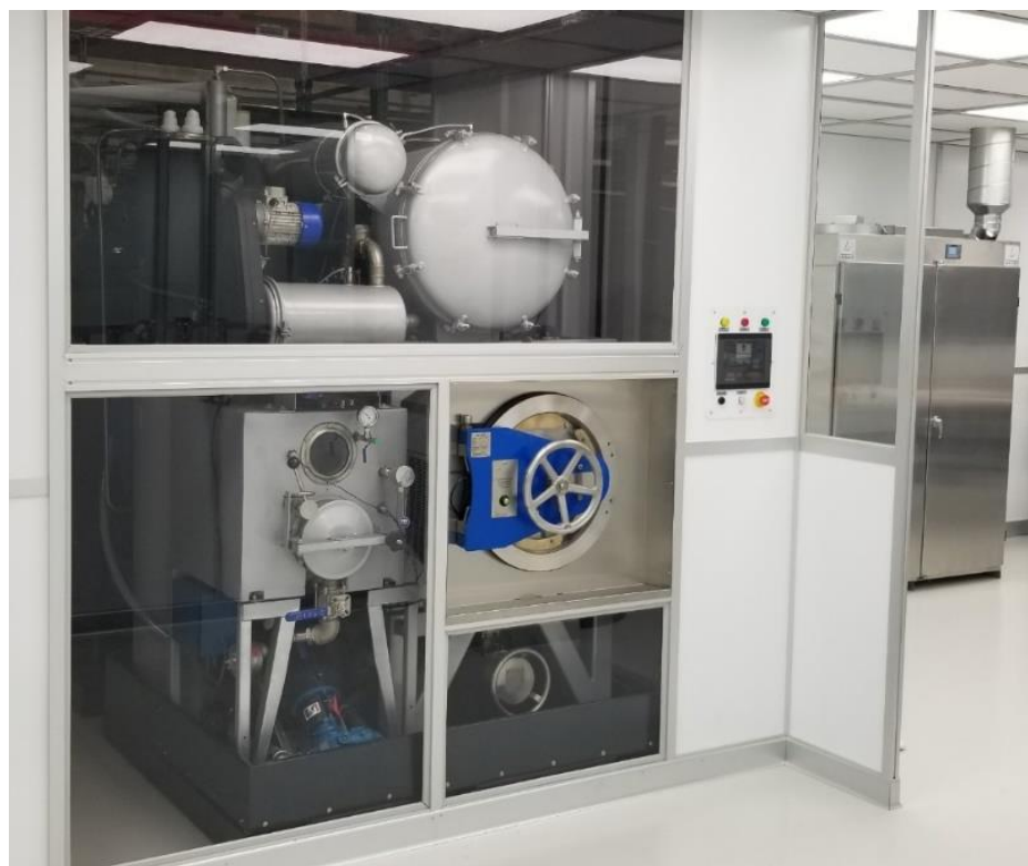
Figure 1 - \text{CO}_2 + Cleaning System located at Emergency Technical Decon – Eagan, MN.
